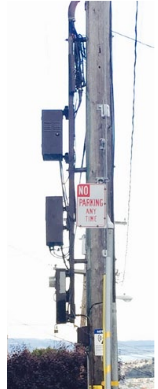
TOP RIGHT: Current Site Photo (after modifications) with disfavored elements such as a wide offset between the pole and equipment enclosures; excess cabling, large bright node identification (yellow placard) and RF warning sticker next to equipment (instead of up near antenna) at pedestrian level.
