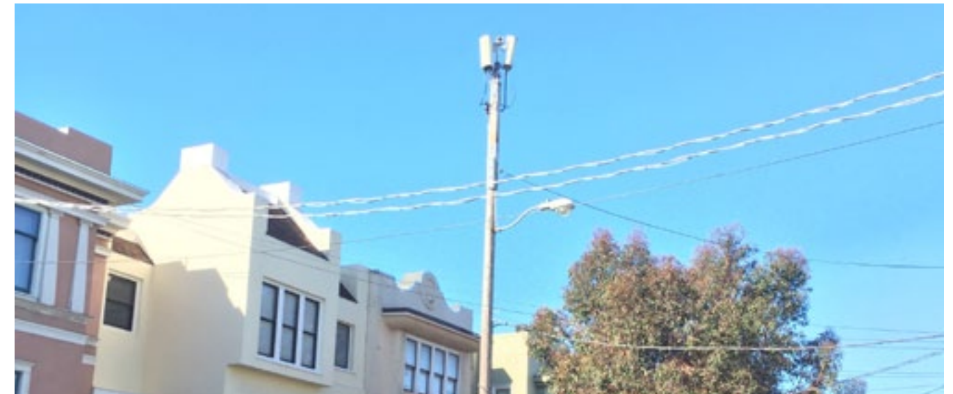
TOP: Disfavored use of multiple panel antennas with wide offset mechanical tilt brackets (evaluate electronic tilt alternatives) and loose cabling
