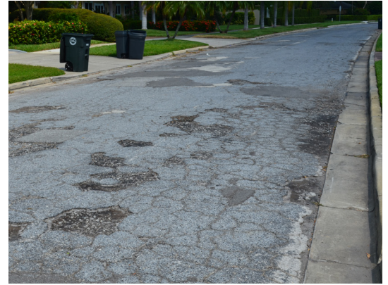
Asphalt degradation along Palmetto Road
