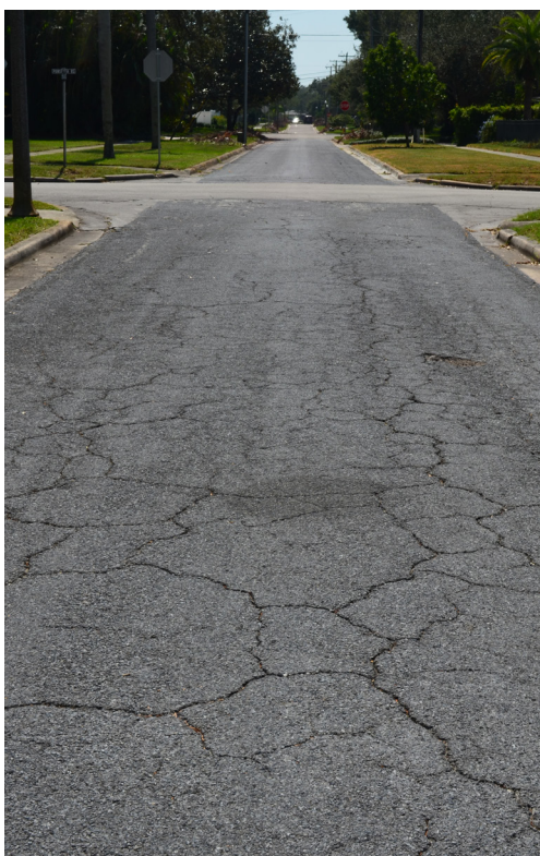
Alligator cracking along Pinellas
