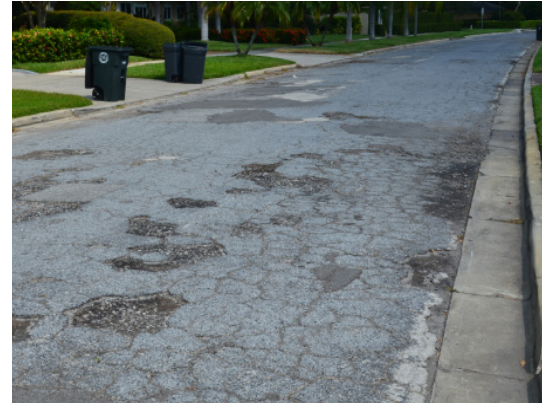
Asphalt degradation along Palmetto Road
