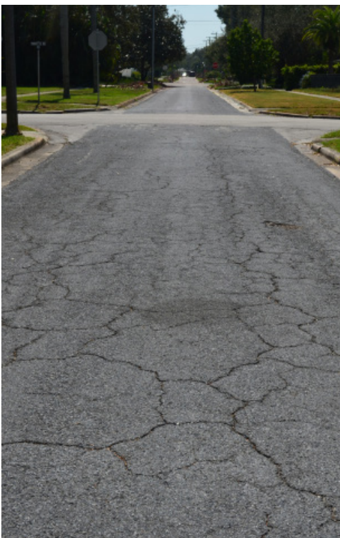
Alligator cracking along Pinellas
