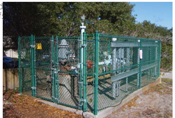
McKim & Creed provided design, construction, testing and analysis of new wells for the City of Clearwater.
