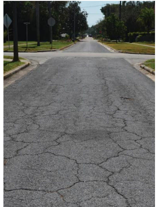
Alligator cracking along Pinellas
