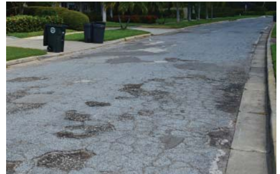
Asphalt degradation along Palmetto Road
