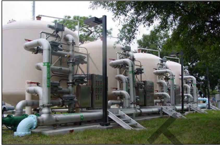
Figure 5-4 – Typical Dual-Media Pressurized Dual-Media Filters, City of Clearwater
